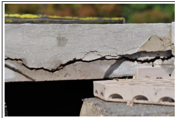
Fig. 7: Typical delaminated Paver.
