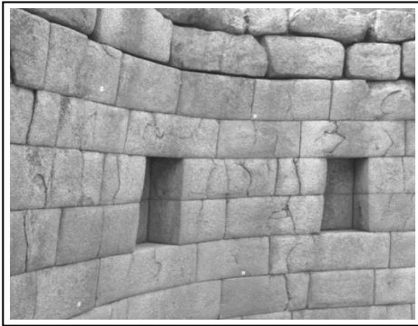
Fig. 5: Cracks and detachments.
