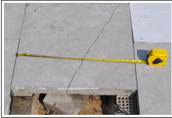
Fig. 1: Typical failed paver.
