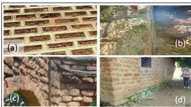
Fig. 4: Views of the most usual defects observed in LDS structures.
